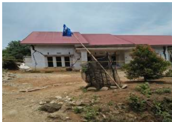
Figure 1. A House Damaged by the Earthquake
