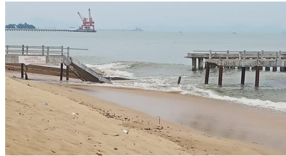
Fig 1. Damage of The Flying Bridge Due to The Impact of Pasir Panjang Beach Abrasion
