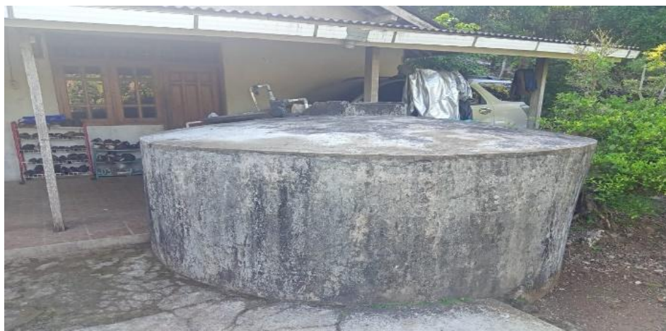
Fig. 2 Rainwater Reservoir (PAH)
